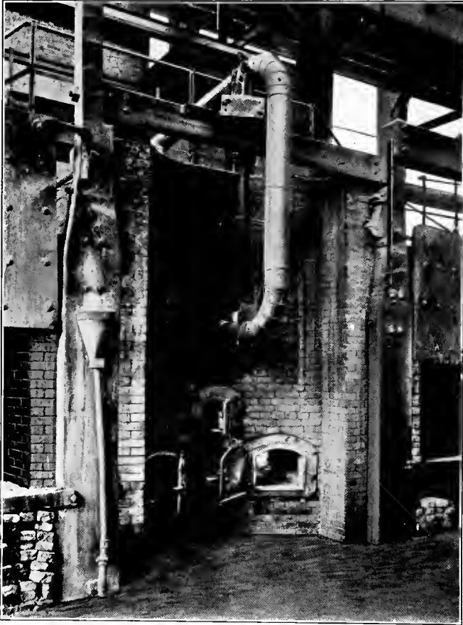
FIG. 101.—Fuller No. 201, Boiler, Fire Box and Burner.
